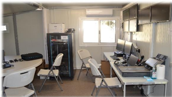
Fig. 6. Interior of the C4I Container and its basic equipment.
